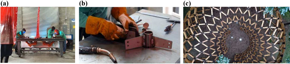
(a) Dual undermounted robotic work-cell used for the fabrication of the 376 welded steel nodes in the Lo-Fab Pavilion (b) Robotic positioning system allows the welder to repeat the same action no matter the node geometry (c) Final assembled pavilion on the Rose Kennedy Greenway in Boston. [Image credits: (a), (b) by Nathan King, Autodesk, (c) by Thatcher Bean, MASS Design Group]
